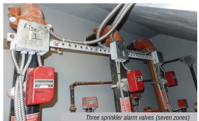
Three sprinkler alarm valves
