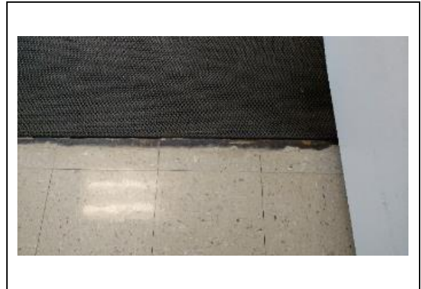
2. Ledge Street School, example of cracked floor tile along the entrance.
