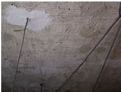
Asbestos Ceiling Plaster
