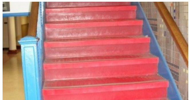
Stairs in original 1936 building do not meet code requirements for dimensions of guardrails, handrails, balusters handrail extensions, etc.
