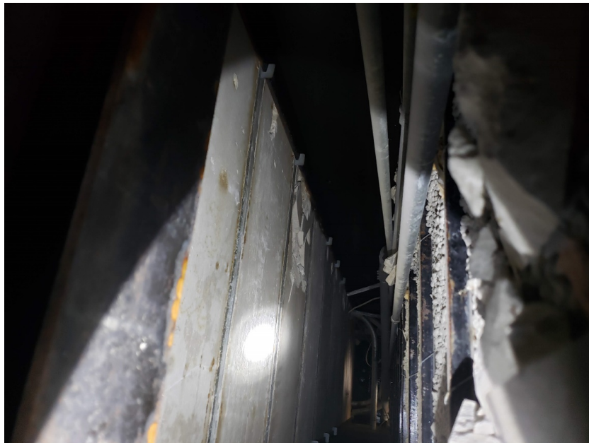
Figure 16 Room 7 Ceiling w/ Spall
