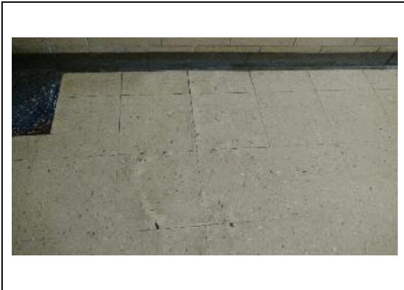
13. Flooring chipped with ACBM Mastic at Main Dunstable.
