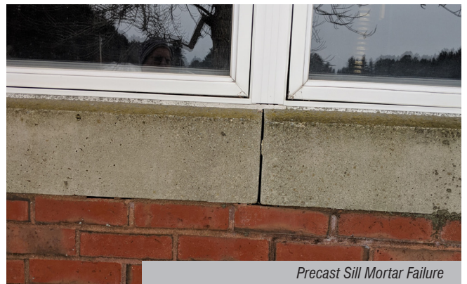
Mortar Spalling- Corner of Gymnasium
