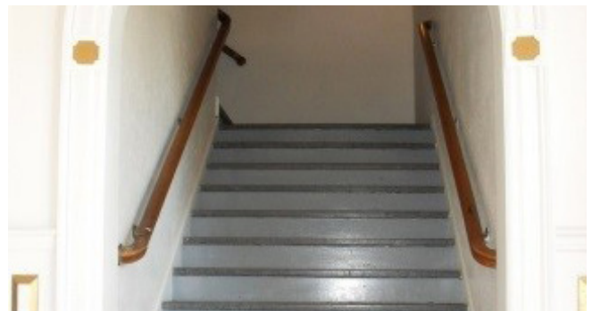
Auditorium Stairs: Access to balcony handrails does not meet code.
