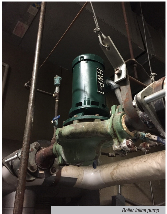
Base mounted pumps
