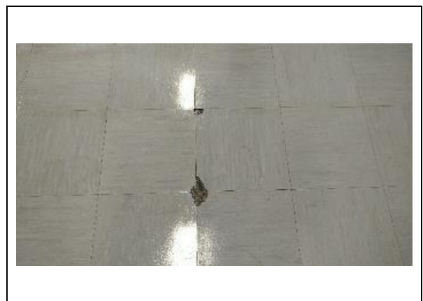
6. Mt. Pleasant, damaged and chipped flooring with mastic exposed.
