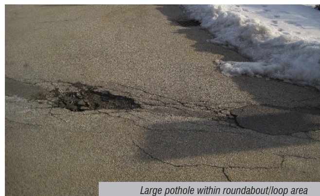
Pavement damage/cracking observed
