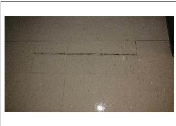
3. Charlotte Avenue, example floor tile damage.
