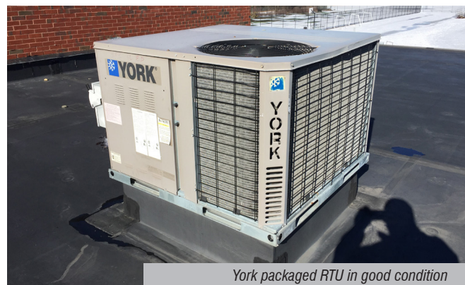
Typical classroom rooftop ventilation unit
