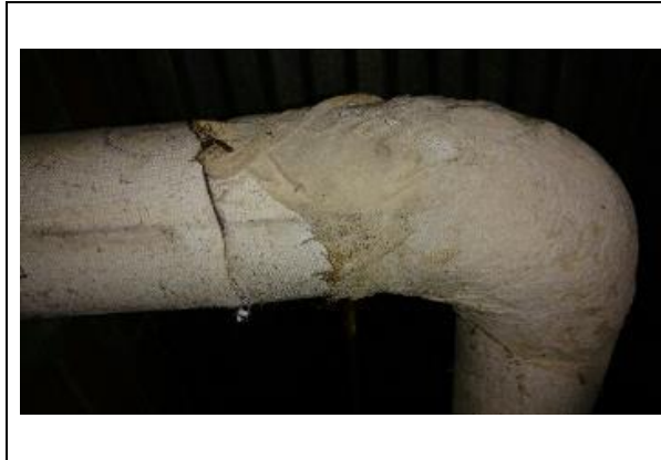
8. Elm Street, damaged pipe fitting outside Room 30 above ceiling.
