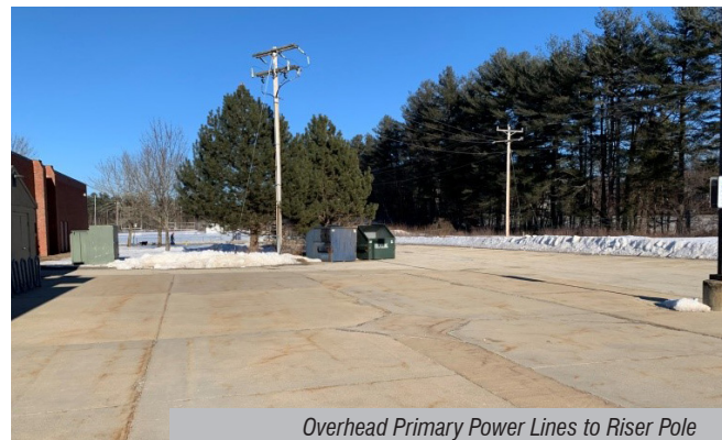
Meter, Portable Generator Connection and Transfer Switch
