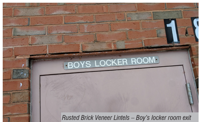
Precast Sill Mortar Failure
