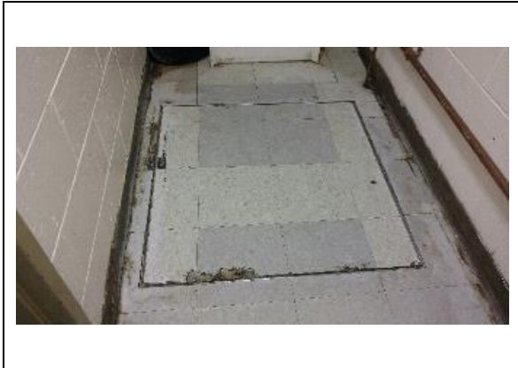
7. Broad Street School, example chipped flooring along a floor hatch with ACBM mastic.
