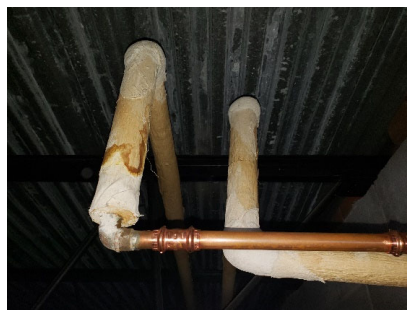
Asbestos Pipe Fittings
