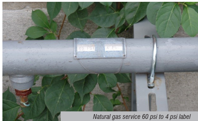
Natural gas service dual pressure regulators
