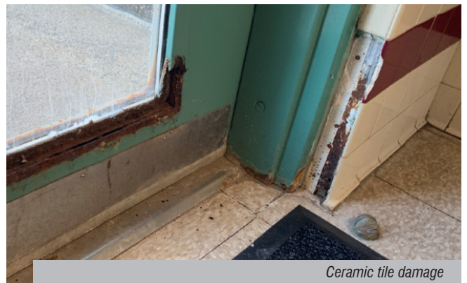
Ceramic tile damage
