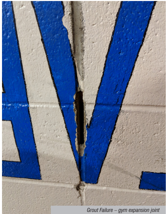
Construction Joint Crack – Cafeteria
