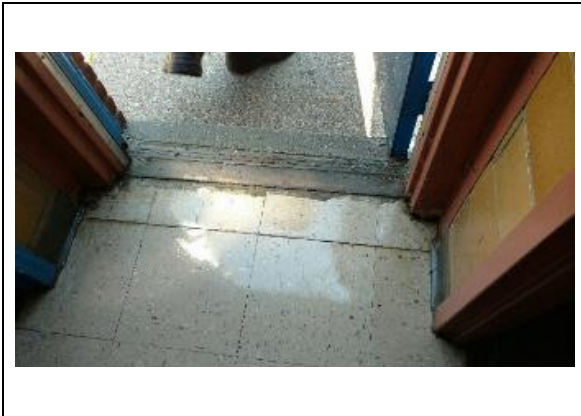
1. Ledge Street School, example of cracked floor tile along the entrance.
