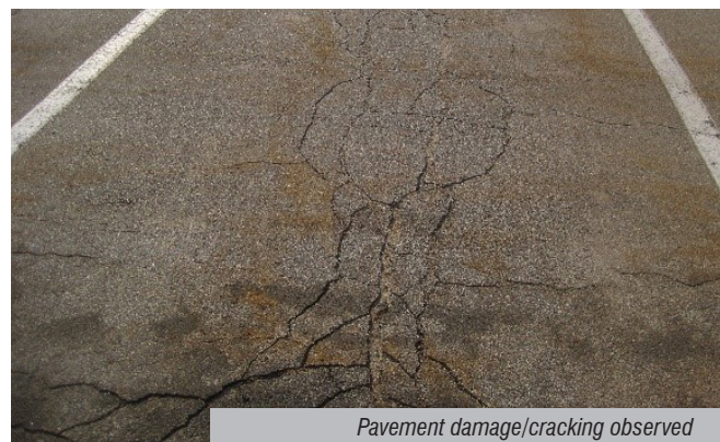
Differential settlement and cracking around manhole
