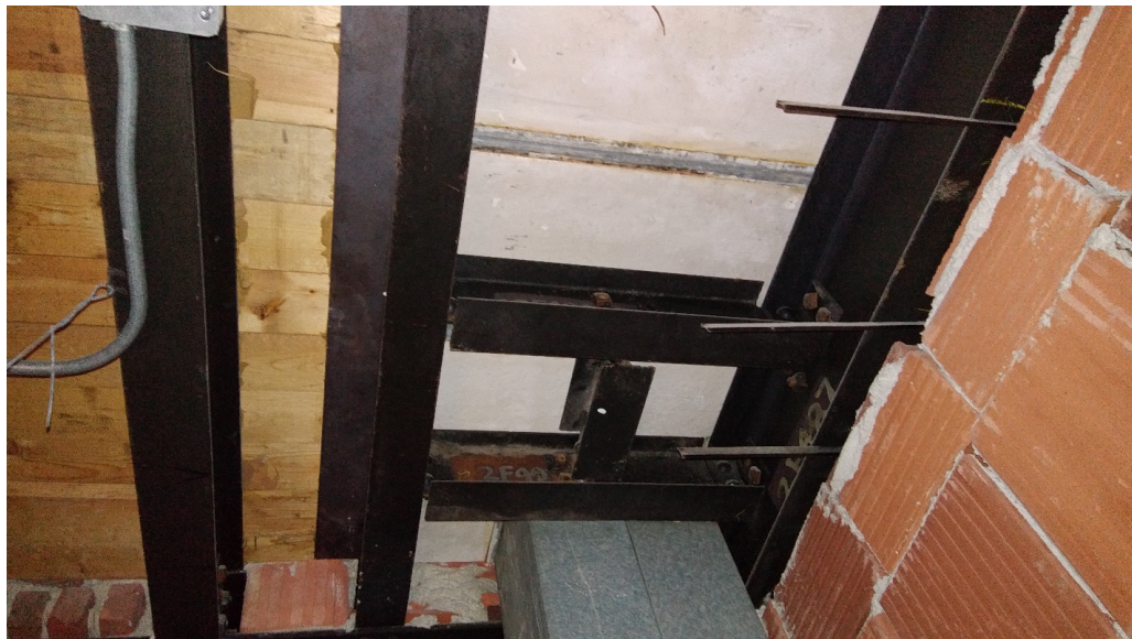
Figure 29 Example of Wood Plank Flooring and Gypsum Panel near Vent Shaft (2 nd floor looking up)
