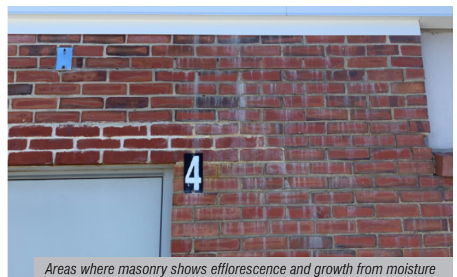
Areas where masonry shows efflorescence and growth from moisture
