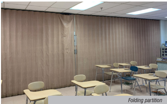
Sagging ceiling tiles in Music
