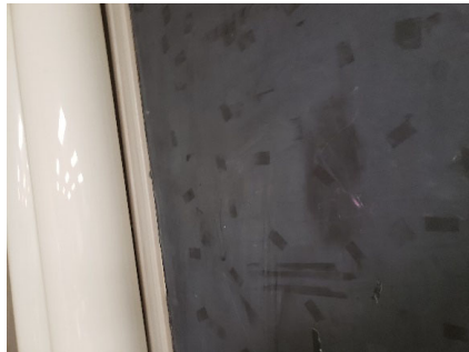
Assumed Asbestos Blackboard
