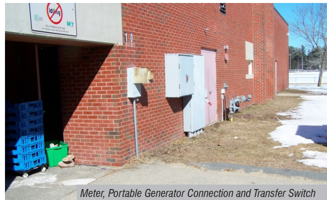
Pad Mounted Transformer – Meter, Portable Generator Connection and Transfer Switch Located on the Building
