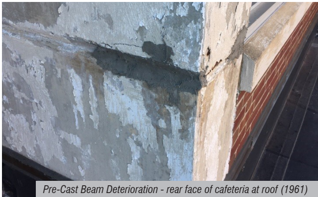
Rusted Lintel and Mortar Damage - east side of industrial arts/STEM wing (1961)
