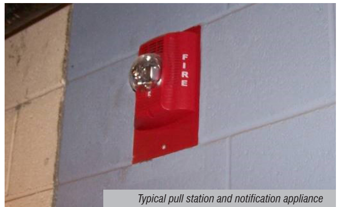
Typical pull station and notification appliance
