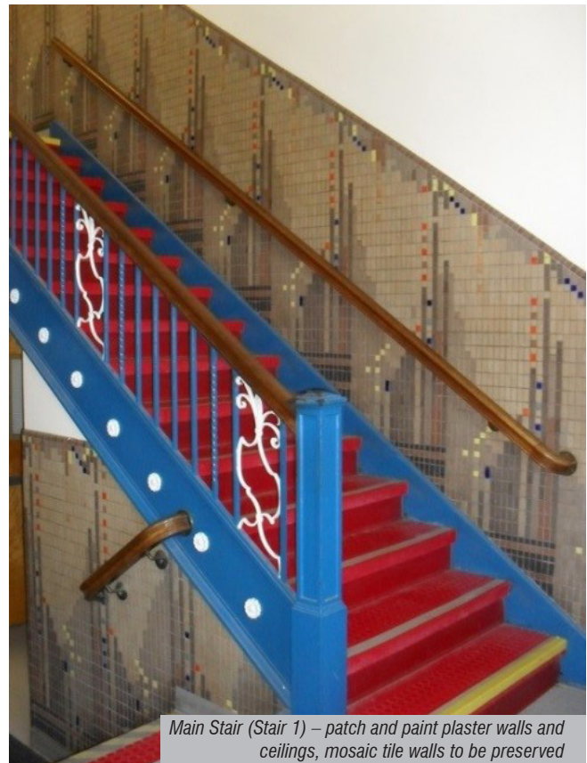
Main Stair (Stair 1) – patch and paint plaster walls and ceilings, mosaic tile walls to be preserved
