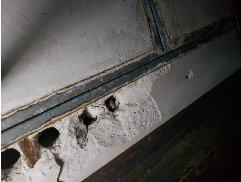
Figure 15 Room 7 Ceiling w/ Drill Holes
