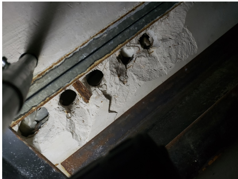
Figure 14 Room 7 Ceiling w/ Drill Holes
