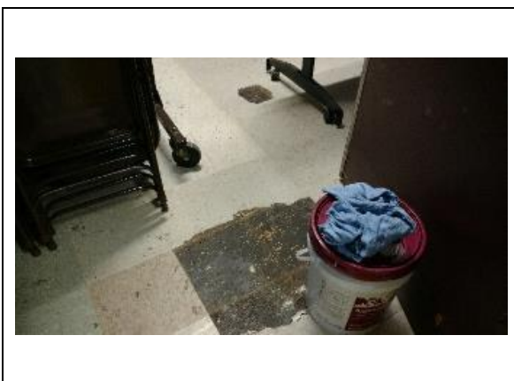
5. Mt. Pleasant, damaged flooring with ACBM mastic exposed in chair room.
