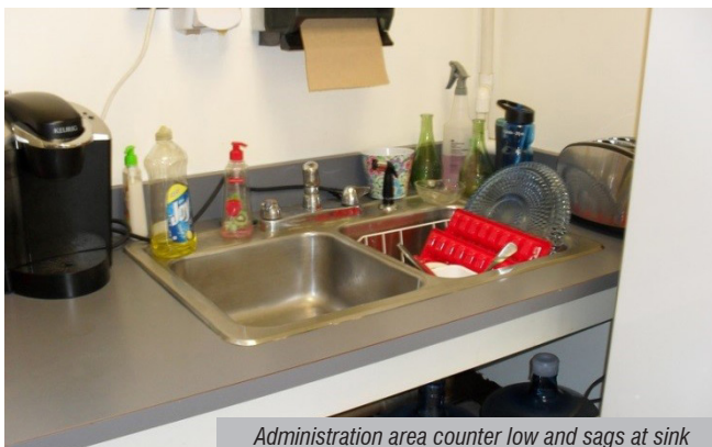
Administration area counter low and sags at sink
