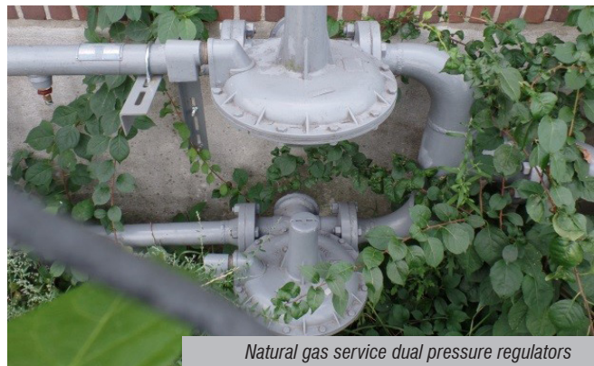
Natural gas service in fenced area
