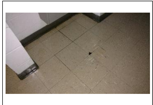
4. Charlotte Avenue, example of flooring damaged.
